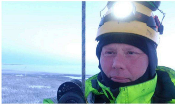
Greger Nilsson from Öjebyn repairs damaged wind turbine blades with an adhesive that hardens in minus degrees. He thinks it is important to emphasize that it is not only foreign companies that work in the wind power industry in northern Sweden.
